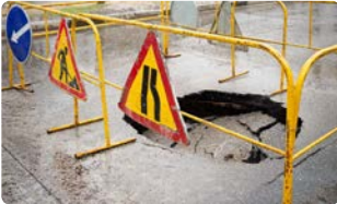
ROAD HAZARD WARNING
