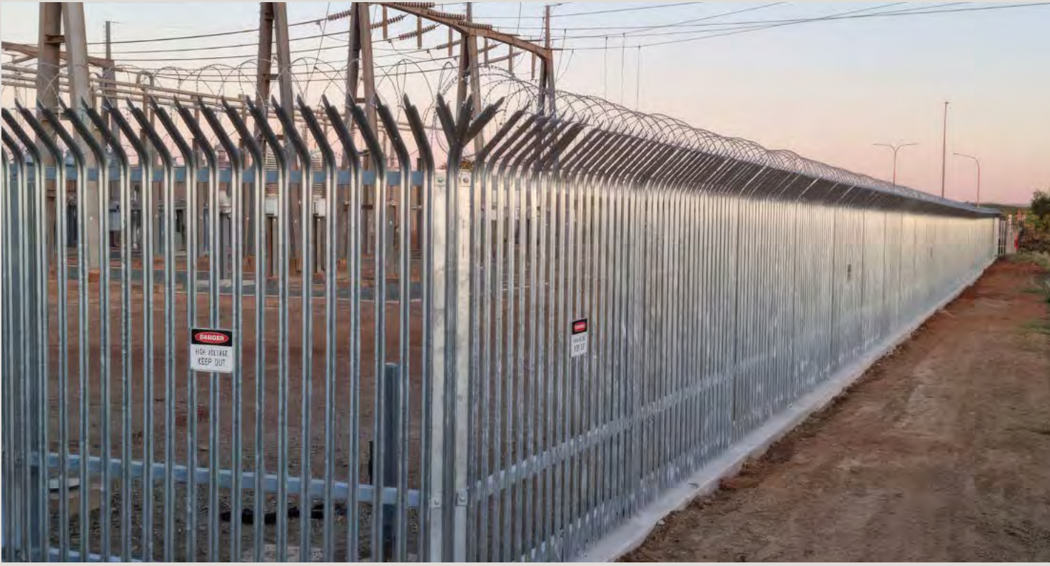
Karratha & Cape Lambert Substations Utilities | WA
