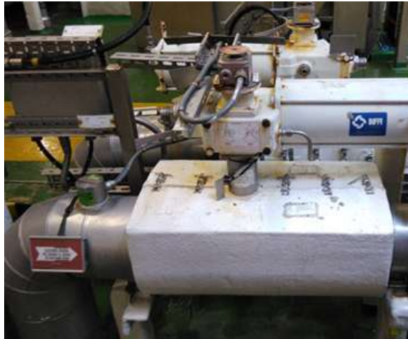
Figure 5 – The 4 inch ball valve closing much faster than both seats and stem is designed for
