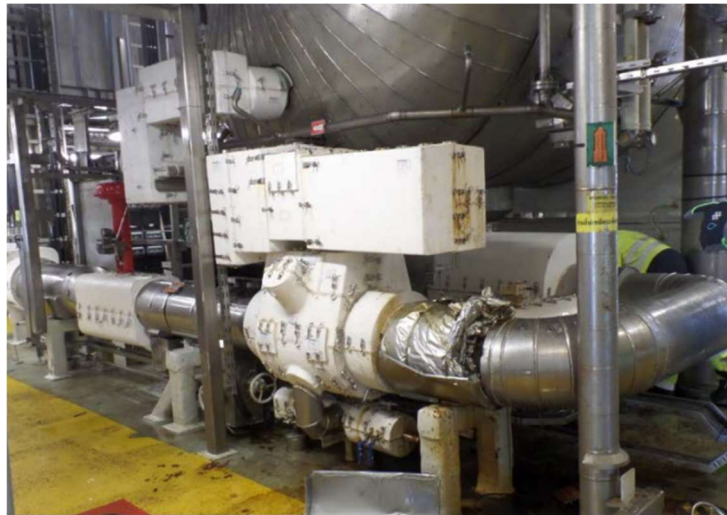
Figure 2 - Emergency Shutdown valve for condensate after 1st stage separator
