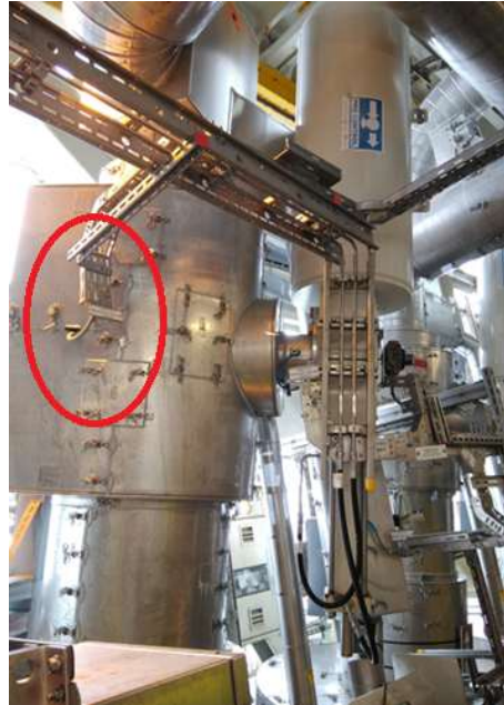
Figure 3 - Insulated water injection valve with acoustic leak sensor.
